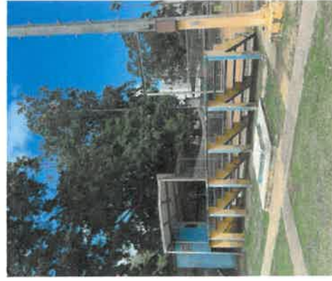
Existing Bleacher's canopy To be repaired.
