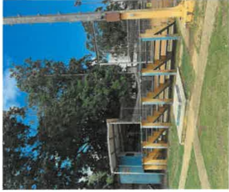
Existing Bleacher's canopy To be repaired.
