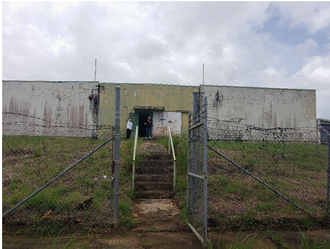
DETERIORATED PAINT 5 SD-04
