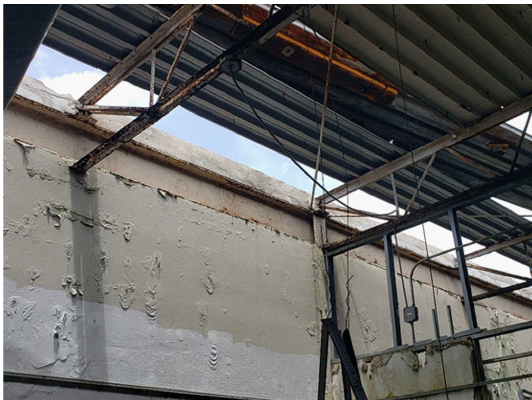
MISSING ROOF DECKING 7 SD-04
