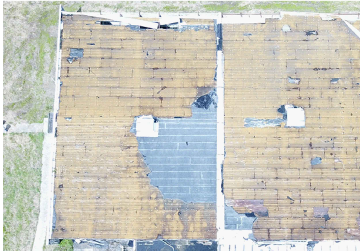
WATERPROOFING AND INSULATION ROOF MEMBRANE DAMAGE 1 SD-04
