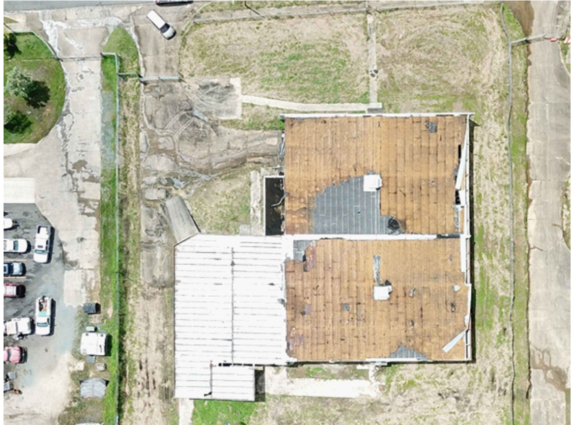
WATERPROOFING AND INSULATION ROOF MEMBRANE DAMAGE 2 SD-04
