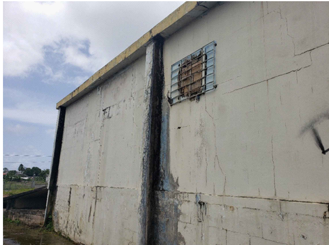
RUSTED COLUMN 6 SD-04
