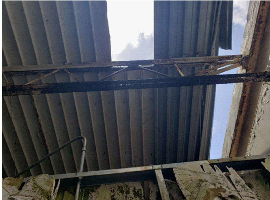
MISSING ROOF DECKING 8 SD-04
