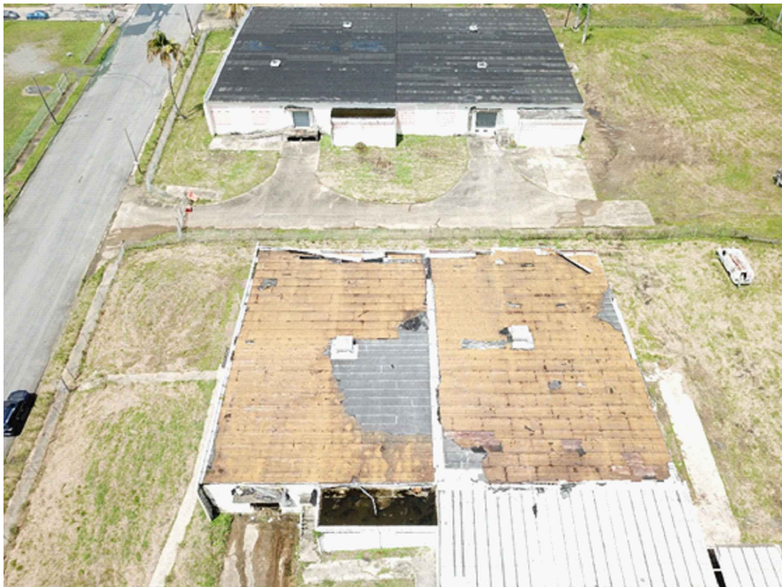
WATERPROOFING AND INSULATION ROOF MEMBRANE DAMAGE 3 SD-04
