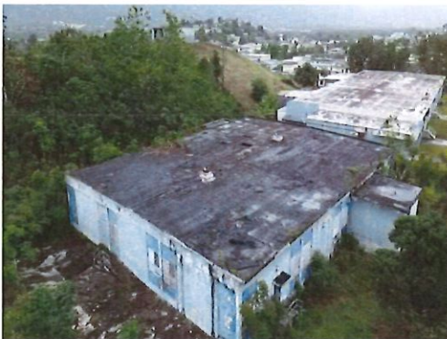
Roofing Materials with Asbestos
