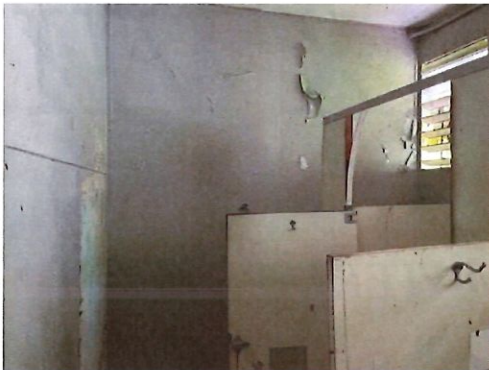
Wall Panel with Asbestos
