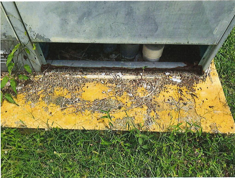
Photo Number 34 – Building Exterior Electric Transformer Slab
