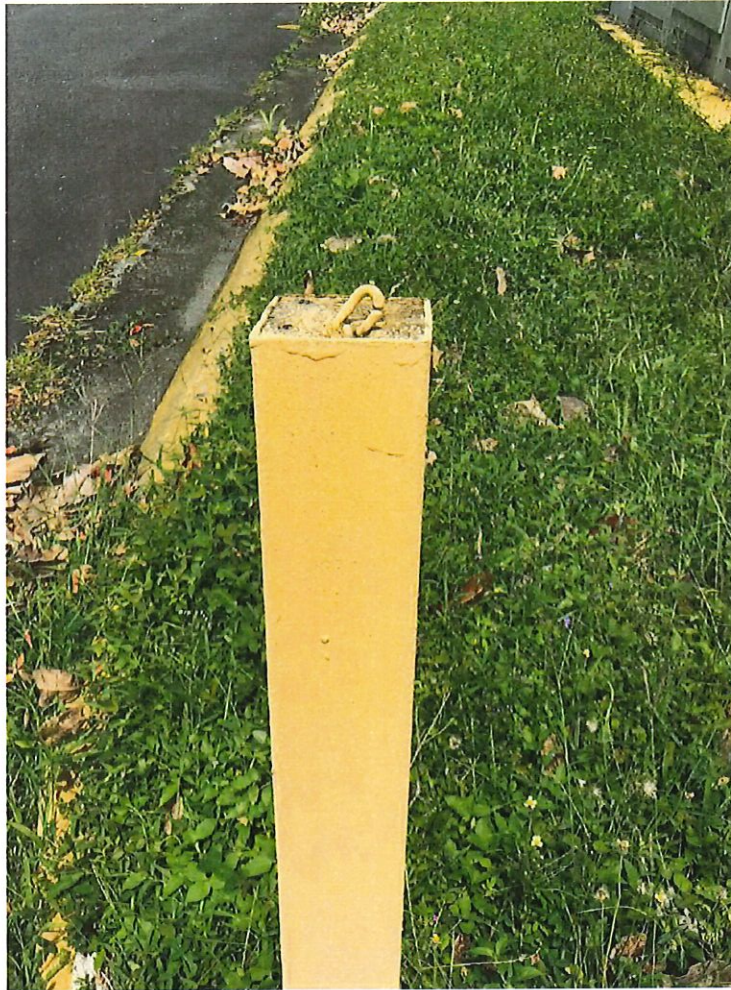
Photo Number 36 – Building Exterior Parking Bollard
