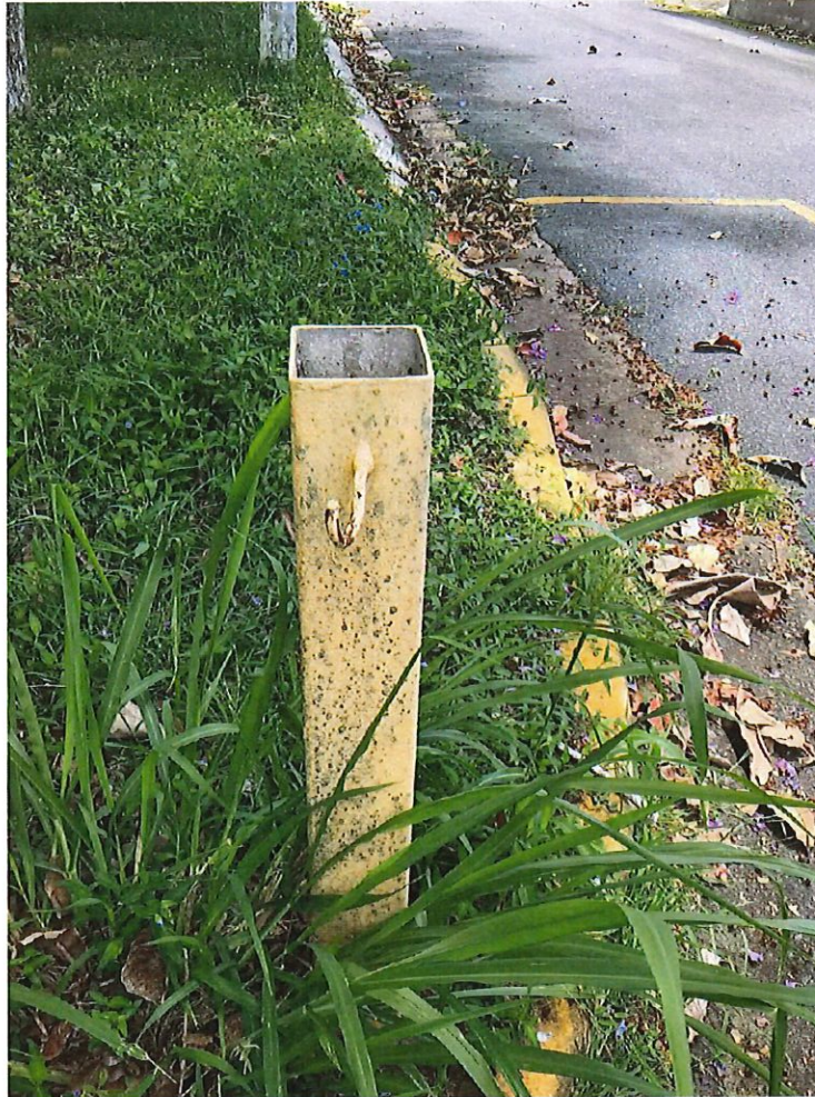
Photo Number 37 – Building Exterior Parking Bollard
