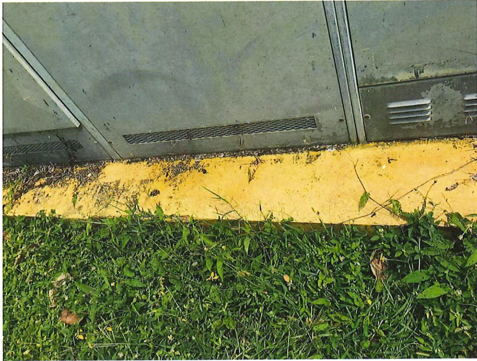
Photo Number 35 – Building Exterior Electric Transformer Slab
