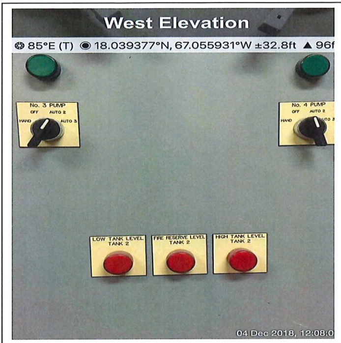
Lajas (CDT) water pump control panel
