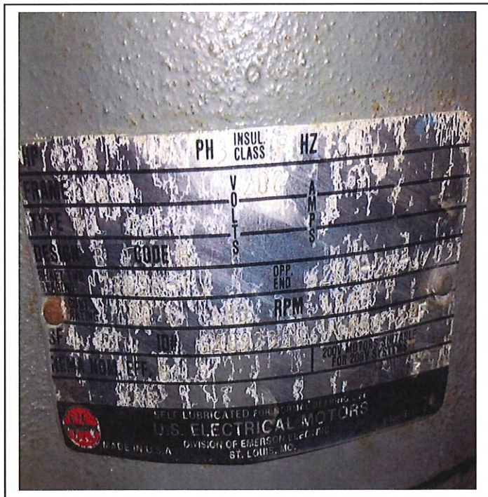
Lajas (CDT) water pump motor tag-pump 4
