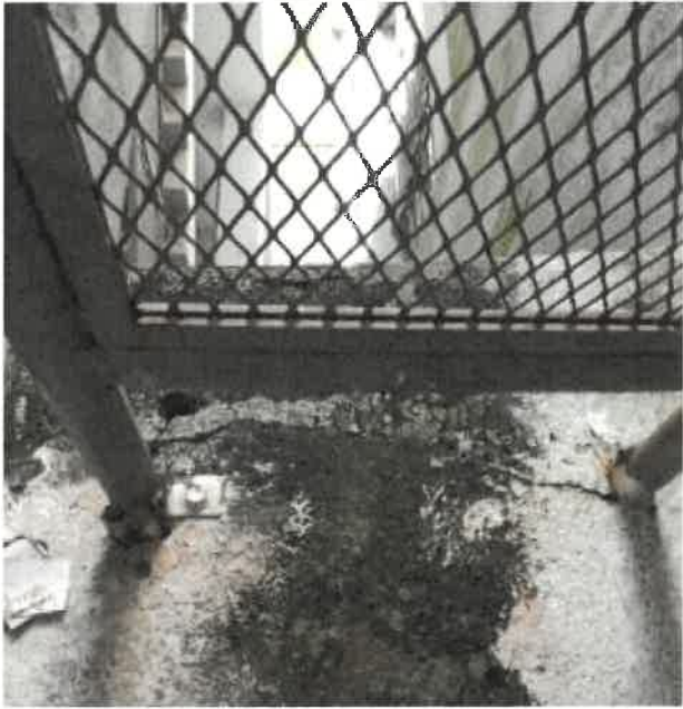
2nd Floor Middle Exterior Stairwell – Concrete Fractures
