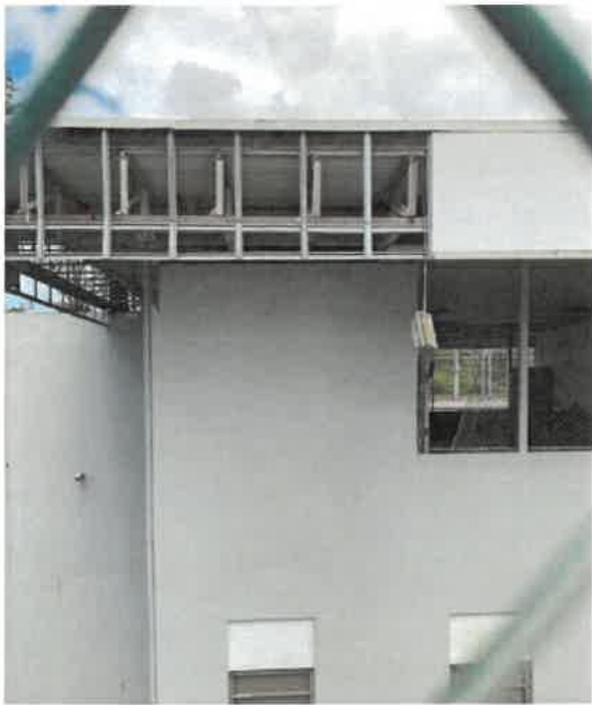
3 rd Floor Roof Covered Area – Soffit & Metal Flashing Destroyed
