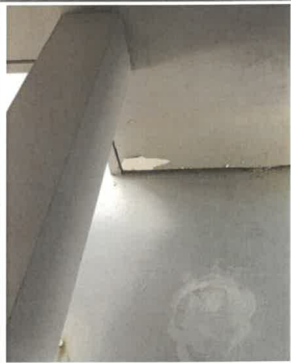
2nd Floor Middle Exterior Stairwell Ceiling – Concrete Fracturing & Detachment From Building Shown
