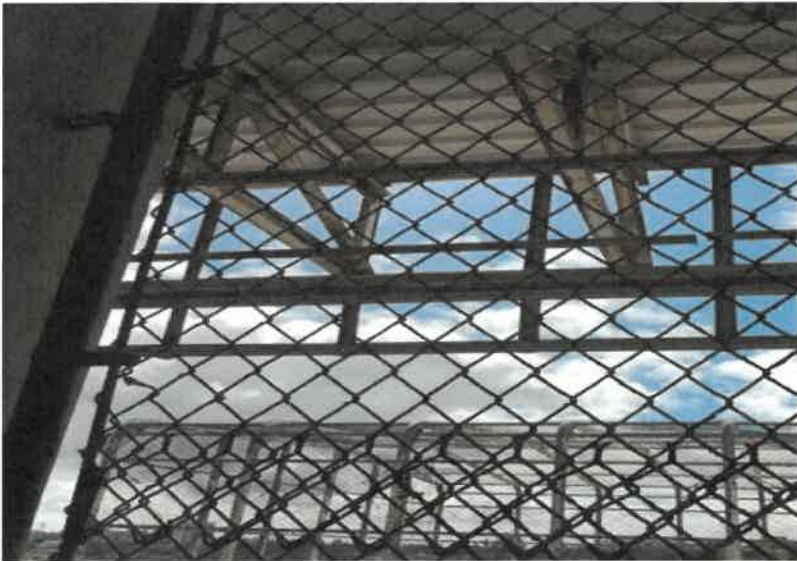
3 rd Floor Roof Covered Area - Damaged/Missing Metal Flashing & Damaged Gypsum Board Ceiling & Soffit
