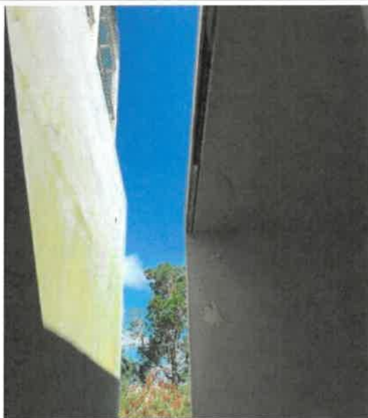
2nd Floor Middle Exterior Stairwell – Exterior Stairwell Concrete Fracturing Visible at 2 nd Floor Ceiling (Shown).
