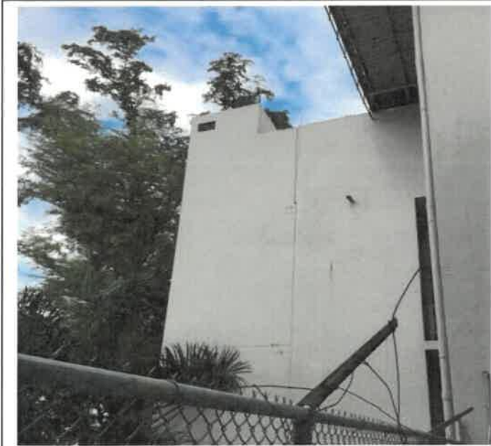
1 st Floor Roof Area – Galvanized Metal Woven Hurricane Fence & Accessories. Damaged Exterior Stairwell in Background.
