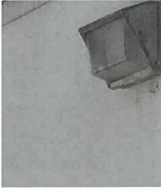
3 rd Floor Roof Covered Area - Close-up Photo of Metal Halide Light Fixture
