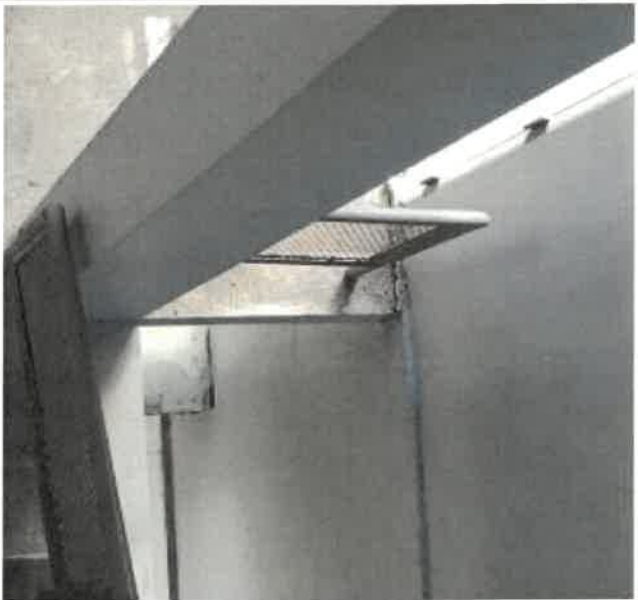
Exterior Stairwell – Photo Vantage is Downward-Looking. Cracked Concrete Visible on First Floor Landing
