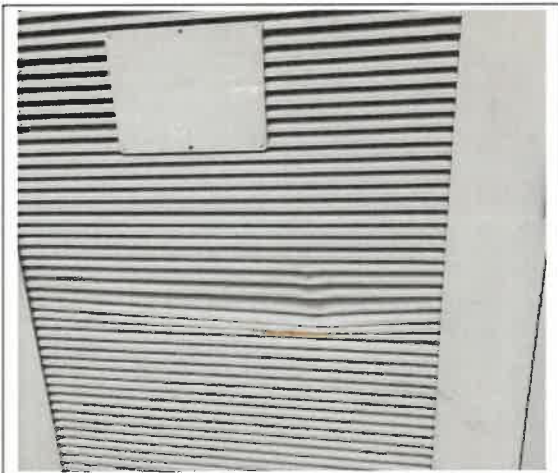
Generator Room - Hollow Metal Louvered Door
