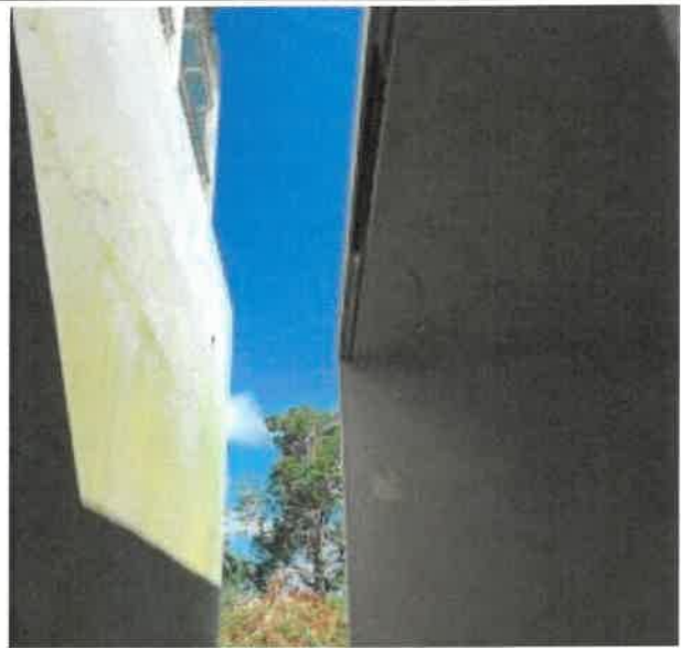
2nd Floor Middle Exterior Stairwell – Exterior Stairwell Concrete Fracturing Visible at 2 nd Floor Ceiling (Shown).
