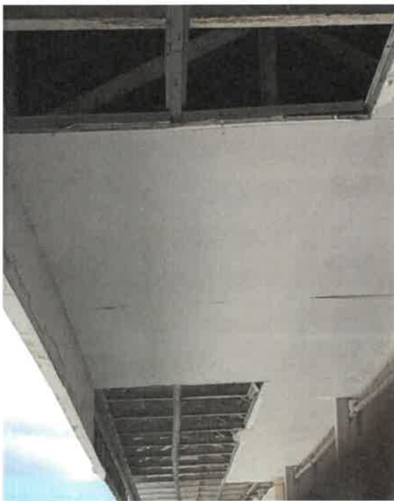
3 rd Floor Roof Covered Area - Damaged/Missing Metal Flashing & Damaged Gypsum Board Ceiling & Soffit
