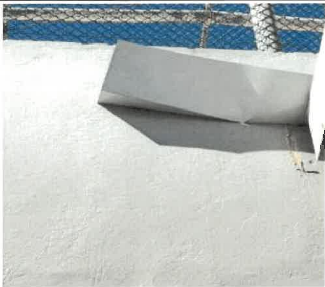
2nd Floor Middle Exterior Stairwell – Exterior Stairwell is Detached From Building. Concrete Fracturing Visible at 2 nd Floor Ceiling (Shown).
