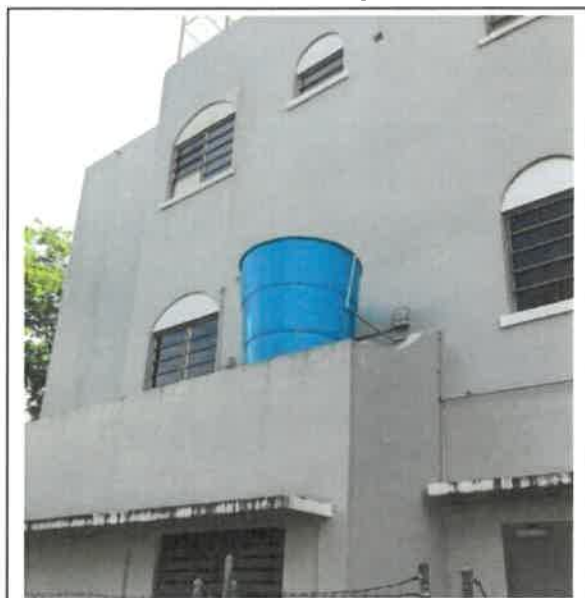
North Building Exterior Mechanical Room Roof - Damaged 600 Gallon Plastic Cistern
