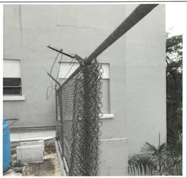
1 st Floor Roof Area – Damaged Hurricane Fence & Accessories
