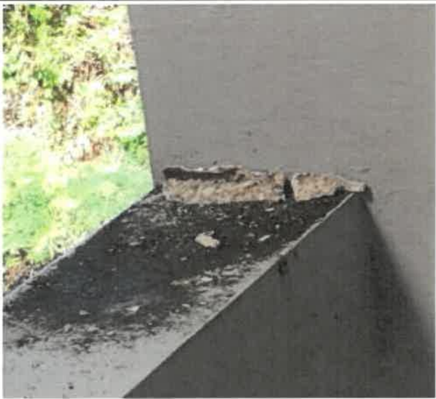
Exterior Stairwell – Concrete Pieces Detached by Tilting/Detachment of Stairwell
