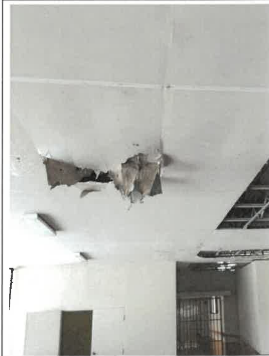
3 rd Floor Roof Covered Area - Damaged Fluorescent Light Fixtures & Damaged Gypsum Board
