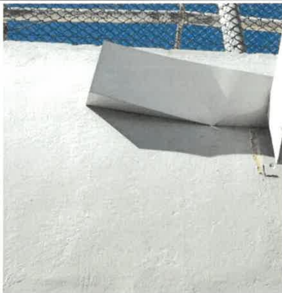
2nd Floor Middle Exterior Stairwell – Exterior Stairwell is Detached From Building. Concrete Fracturing Visible at 2 nd Floor Ceiling (Shown).
