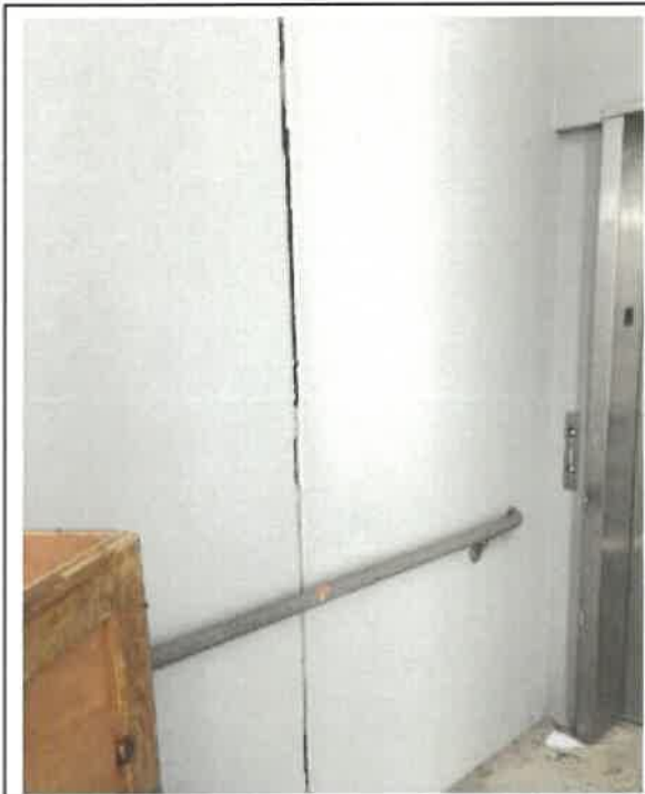
2nd Floor Middle Exterior Stairwell – Detachment of Elevator Shaft Structure From Exterior Stairwell Shown
