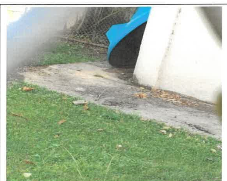
North Building Exterior Mechanical Room Roof Cistern - Damaged 600 Gallon Plastic Cistern
