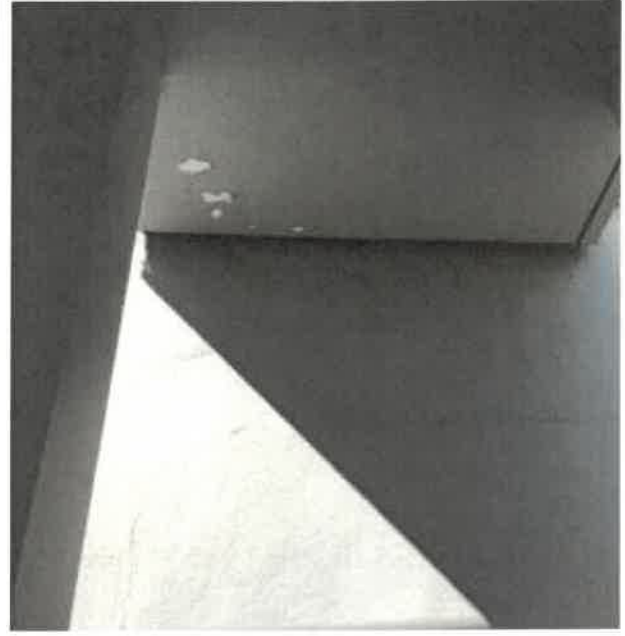
2nd Floor Middle Exterior Stairwell – Exterior Stairwell is Detached From Building. Concrete Fracturing Visible at 2 nd Floor Ceiling (Shown).
