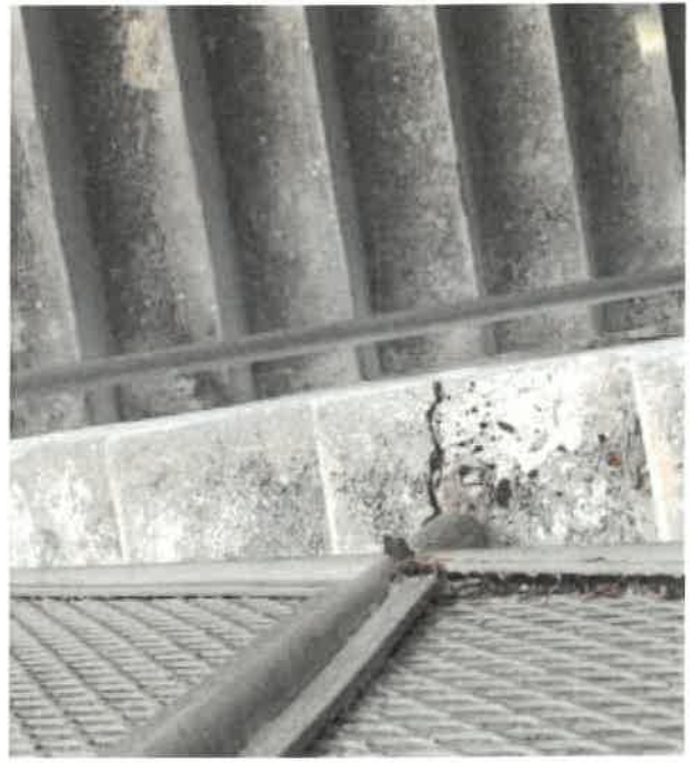
2nd Floor Middle Exterior Stairwell – Concrete Fracturing Visible at 2 nd Floor Steps (Shown).
