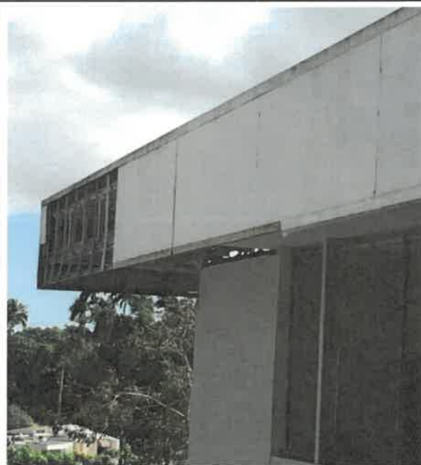
3 rd Floor Roof Covered Area – Damaged Gypsum Board & Damaged/Missing Metal Flashing
