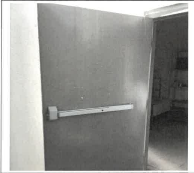
NW Exterior Ground Level – Hollow Metal Door in Need of Realignment
