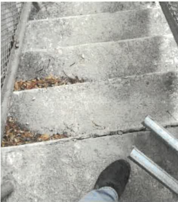
2nd Floor Middle Exterior Stairwell – Concrete Fracturing Visible at 2 nd Floor Steps (Shown).
