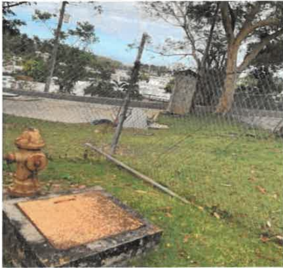
Facility Perimeter - Galvanized Metal Woven Hurricane Fence With Accessories
