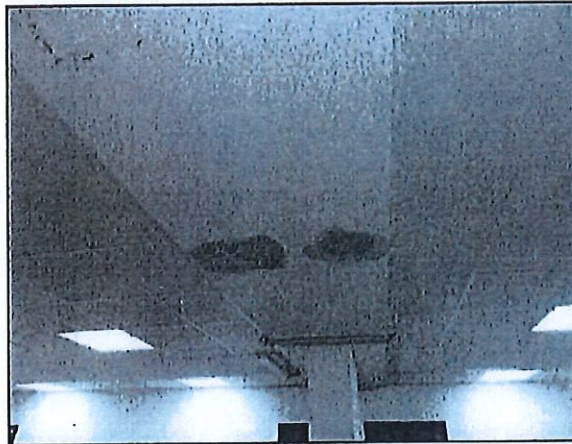
Asbestos Containing Spray-on Ceiling Finish
