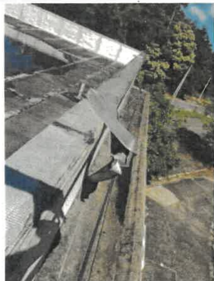
Photo 47 – Damaged 10 FT roof parapet wall section, bended and broken
