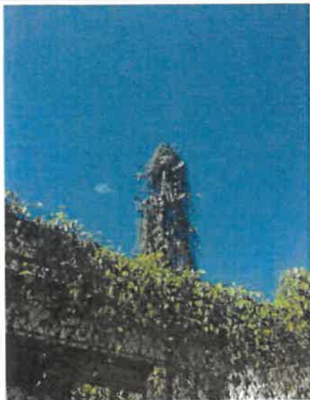
Photo 61 – Damaged electrical utility pole (40 FT height)
