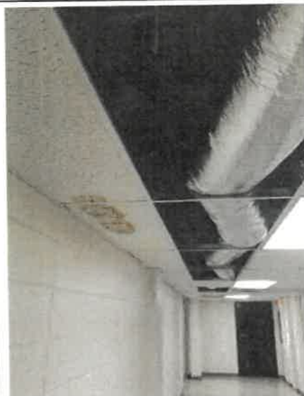
Photo 18 – Hallway behind Pharmacy Area (south side), damaged acoustic tiles (2 FT wide by 4 FT height)
