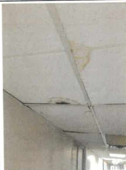
Photo 20 – Hallway continuation from Lobby (east side), damaged acoustic tiles (2 FT wide by 4 FT height)
