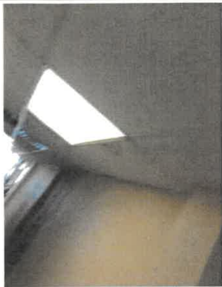
Photo 21 – Hallway continuation from Lobby (east side), damaged acoustic tiles (2 FT wide by 4 FT height)
