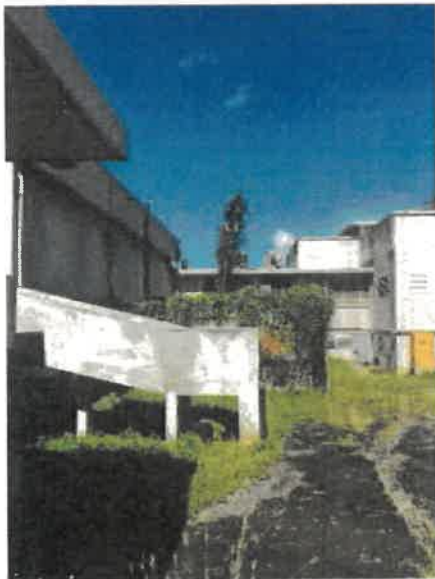
Photo 59 – Damaged electrical utility pole (40 FT height)
