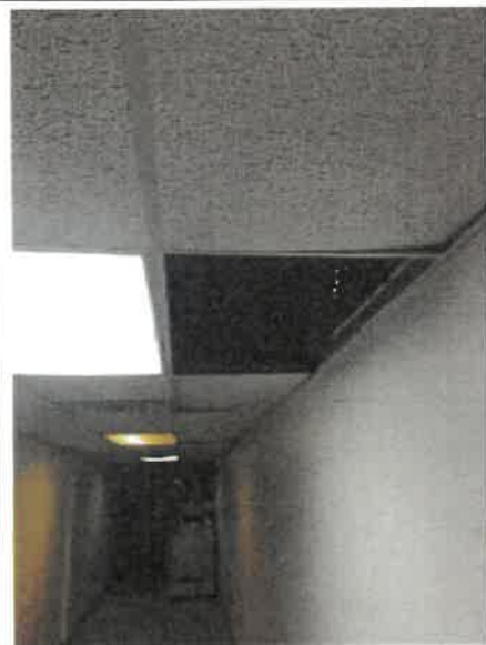
Photo 23 – Hallway, OCASET, damaged acoustic tiles (2 FT wide by 4 FT height)
