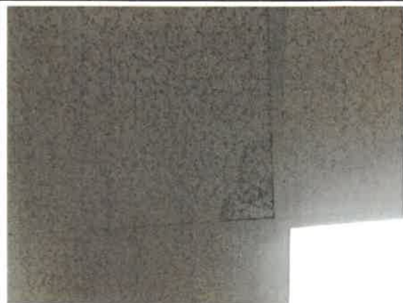
Photo 30 – VIH Monitoring Office, damaged acoustic tiles (2 FT wide by 4 FT height)
