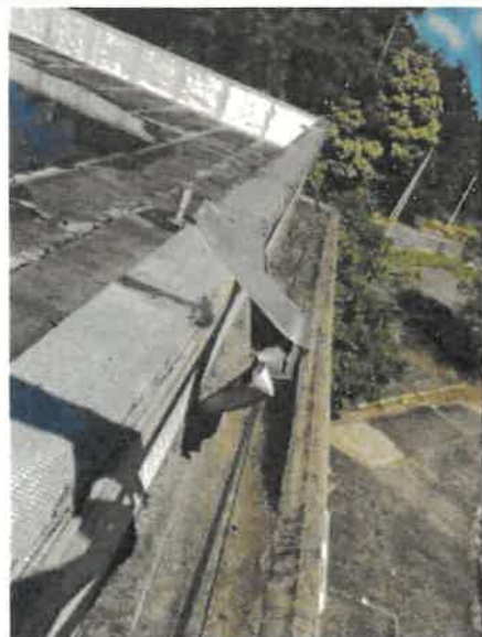
Photo 47 – Damaged 10 FT roof parapet wall section, bended and broken
