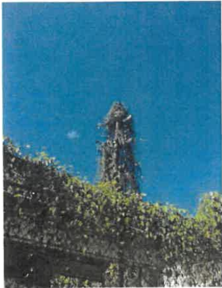
Photo 61 – Damaged electrical utility pole (40 FT height)
